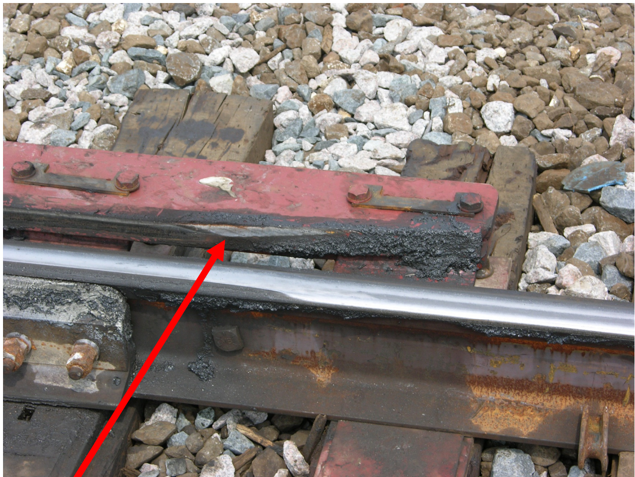
Heavy wear on switch point protector
